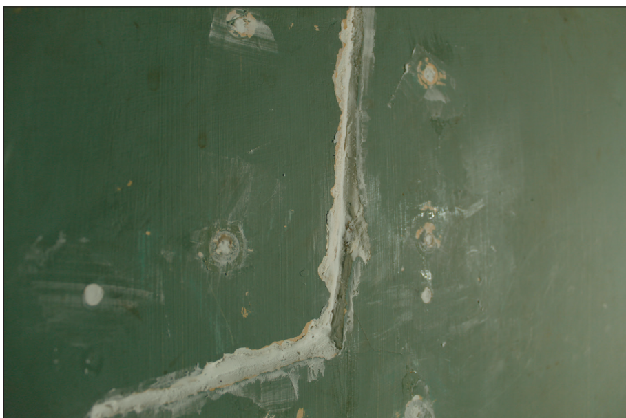
We used spackle as the first layer in this deeper part of the crack, figuring it would be rough enough for the next—plaster—layer to stick on.
